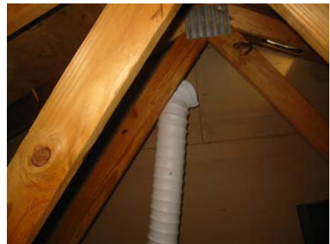
BATHROOM EXHAUST VENT TERMINATES IN ATTIC RATHER THAN OUTSIDE
