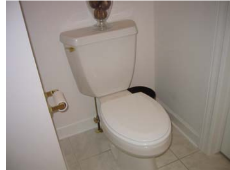
TOILET IN MASTER BATHROOM IS LOOSE AT BASE, SEAL LEAKING
