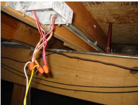
EXPOSED HIGH VOLTAGE WIRING OPEN JUNCTION BOX AT BASEMENT CEILING
