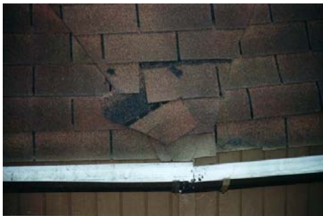
ROOF SHINGLES DAMAGED AT GARAGE REAR ELEVATION
