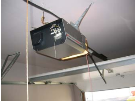
SAFETY REVERSE AT GARAGE DOOR NOT FUNCTIONAL
