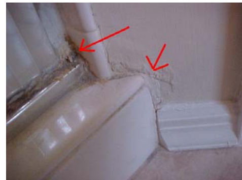
WATER LEAK AND WALL DAMAGE AT HALLWAY BATHROOM SHOWER BASE
