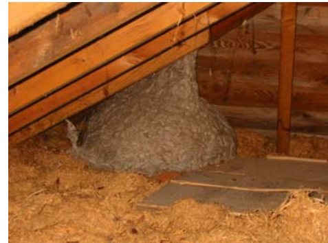
LARGE HORNETS NEST LOCATED IN ATTIC
